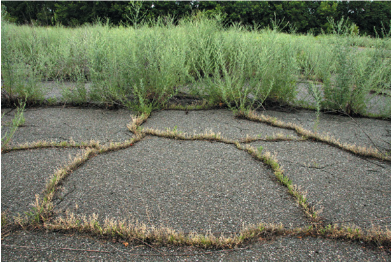
Urban vegetation takes hold in cracks in a neglected swath of asphalt pavement.
